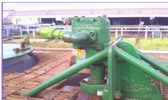
Gambar IV.4 Valves (Sumber: PT. Shinkobe Engineering, 2016)
