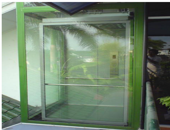
Gambar IV.5 Freight & Hospital Elevator ( Sumber: PT Rekayasa Mitra Mandiri )
