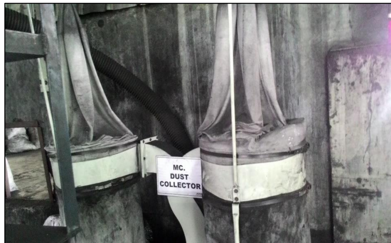
Gambar IV.9 Mesin Dust Collector (Sumber: PT Nandya Briket Brata, 2016)
