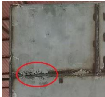
Gambar 4. 13 Cacat Incomplete Penetration (Sumber: PT Astanita Sukses Apindo)
