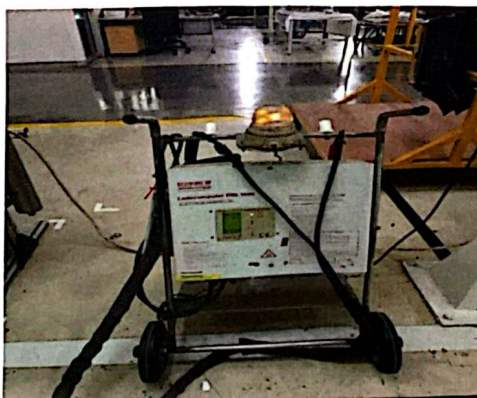
Gambar 4.8. Charger Battery (Sumber: PT XYZ Indonesia)
