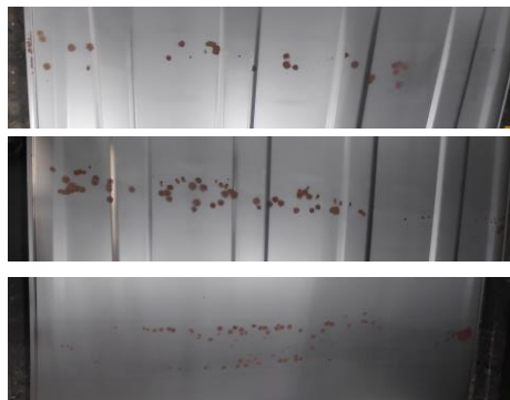
Gambar 4.12 Defect Rust Part Panel Roof (Sumber: PT TMMIN)
