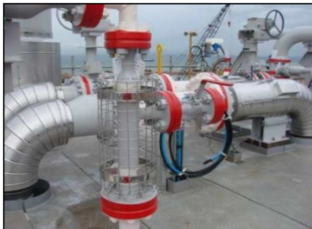
Gambar 4.1 Equipment and Pipe Thermal Insulation Sumber: PT Krazu Nusantara
